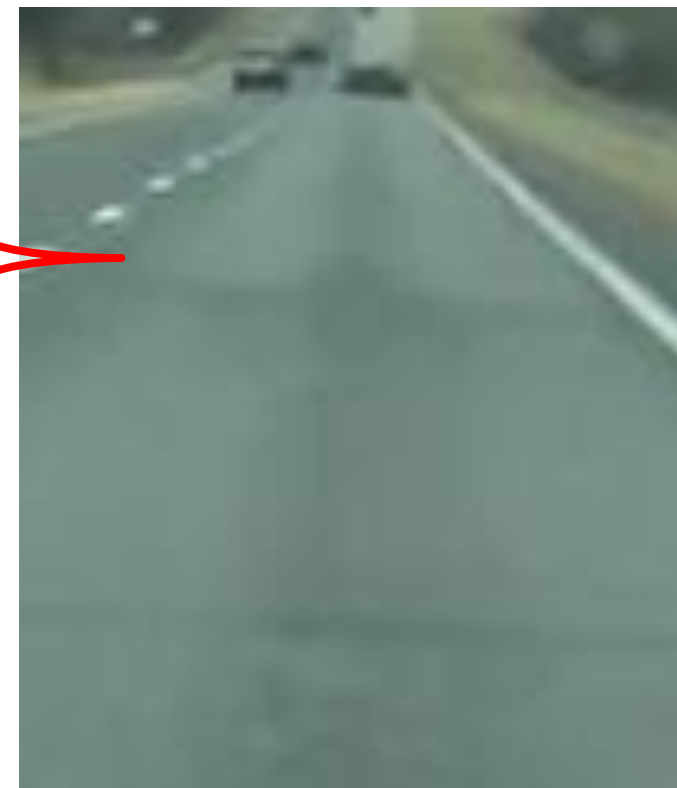
Raveling - Premature Failure
