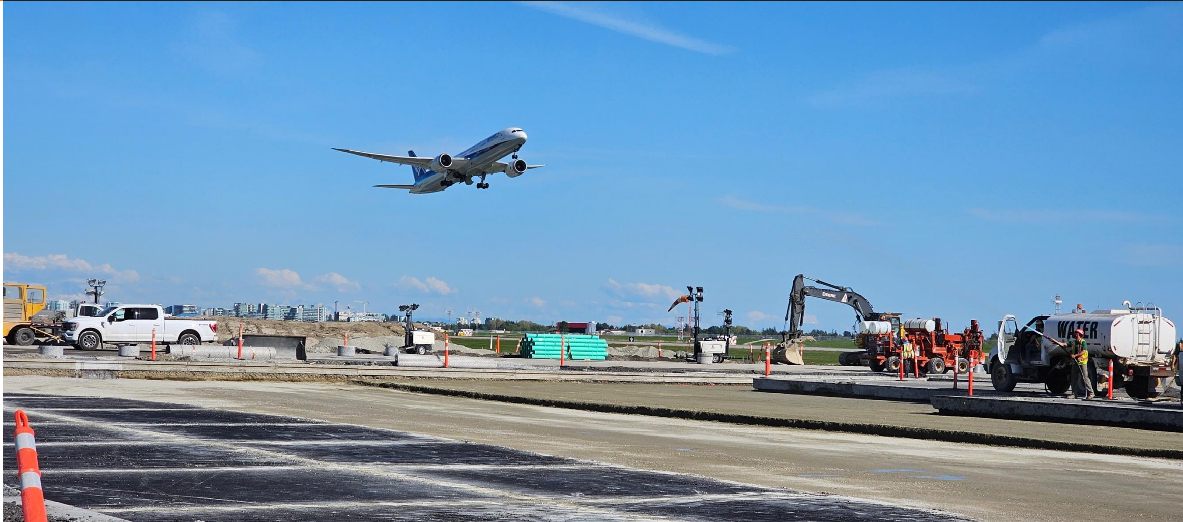
YVR International Airport South Airfield Pavement Rehabilitation 2023 (Taxiway L, L2, L4, L6, D3)
