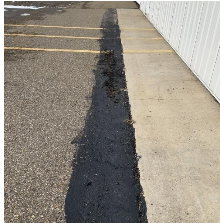
Ramping patch in poor condition
