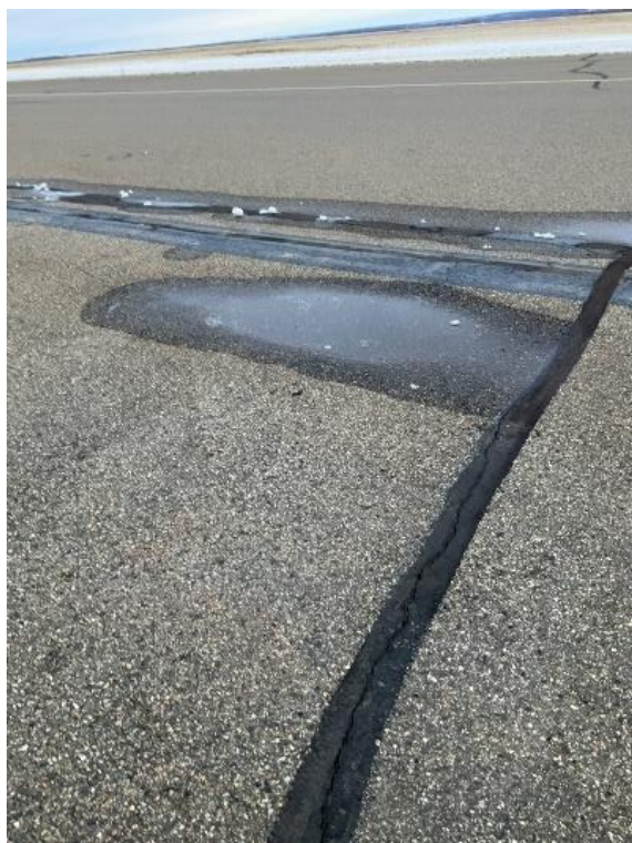
Cracks w/ poor sealant and depression
