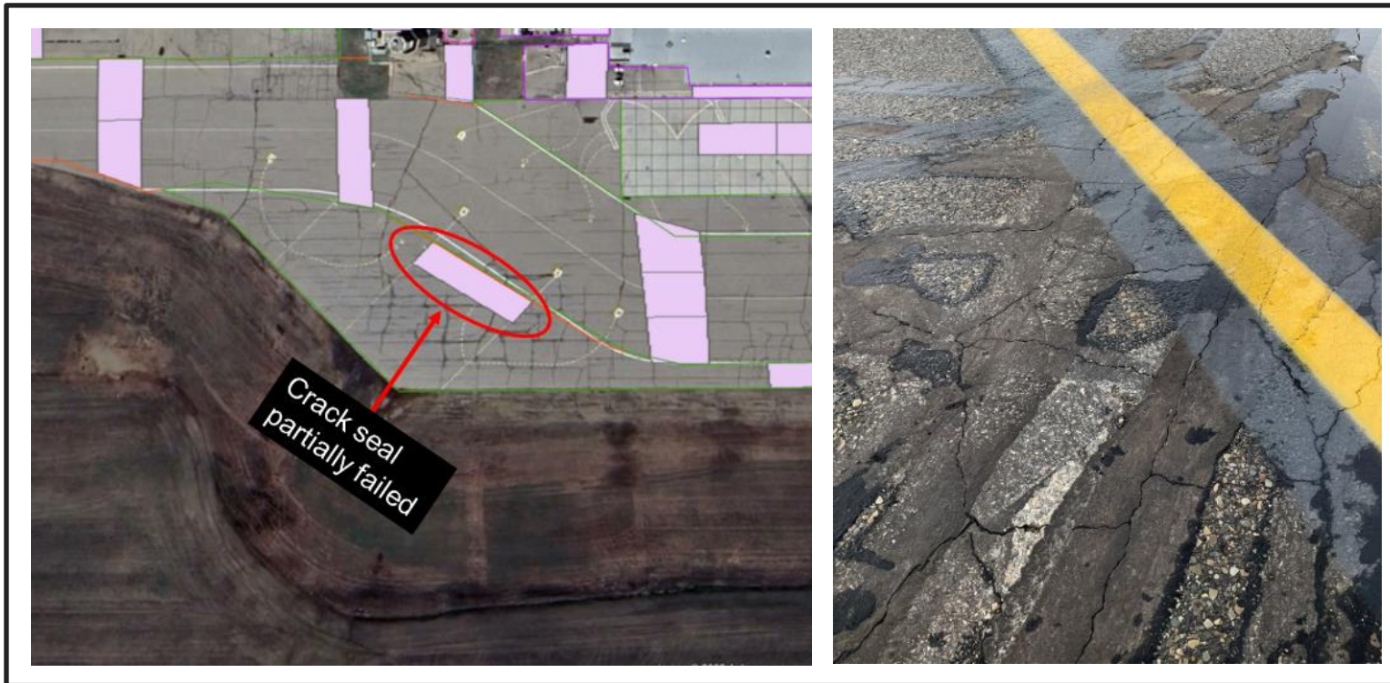
Sealed cracks, some partially failed
