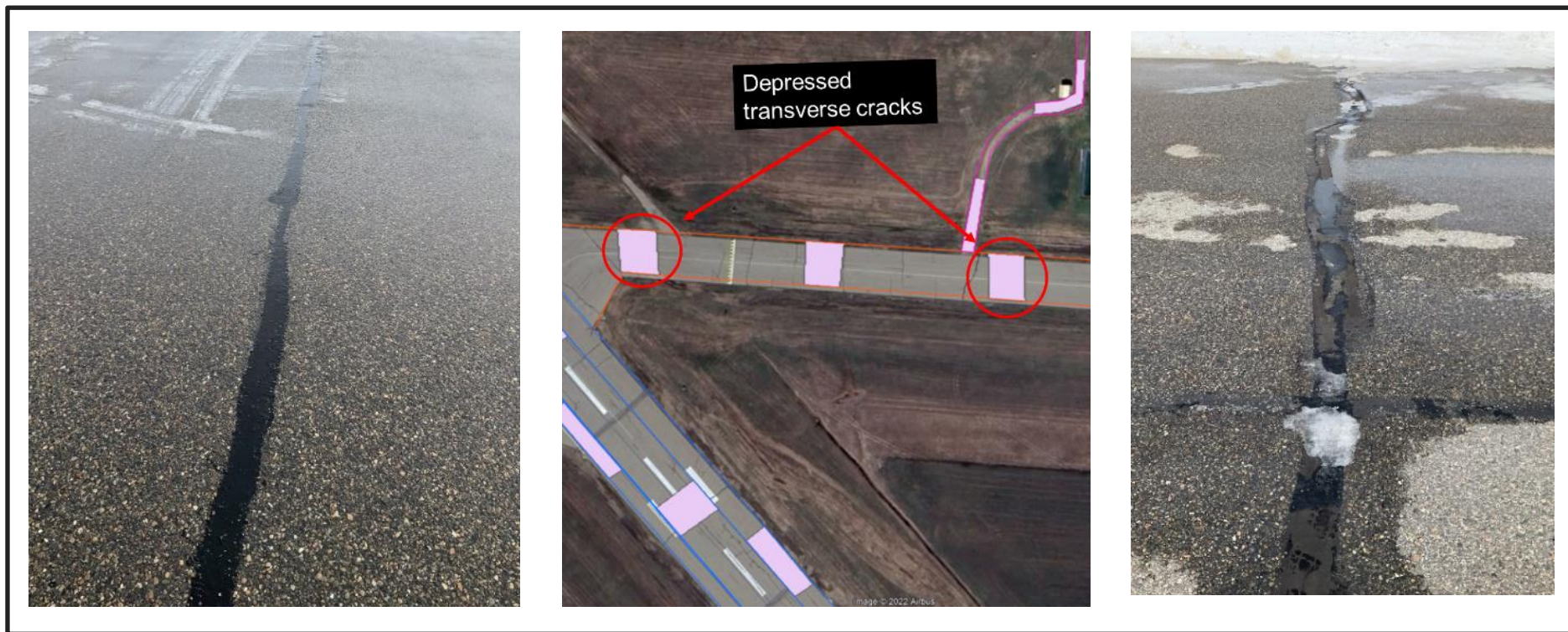
Cracks sealed, mostly in good condition
