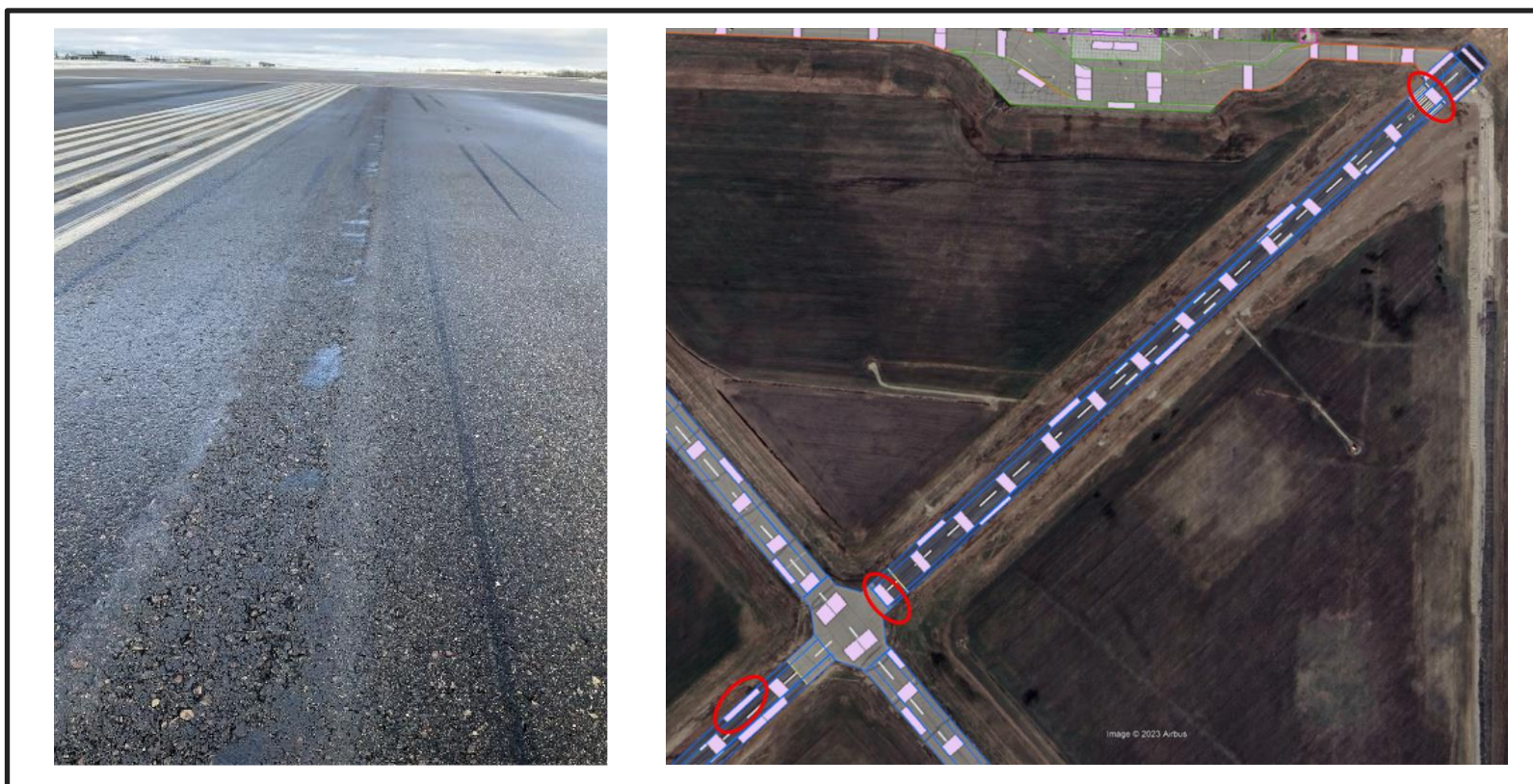
Mild Weathering and Raveling
