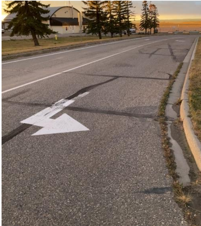
Edge cracking with vegetation
