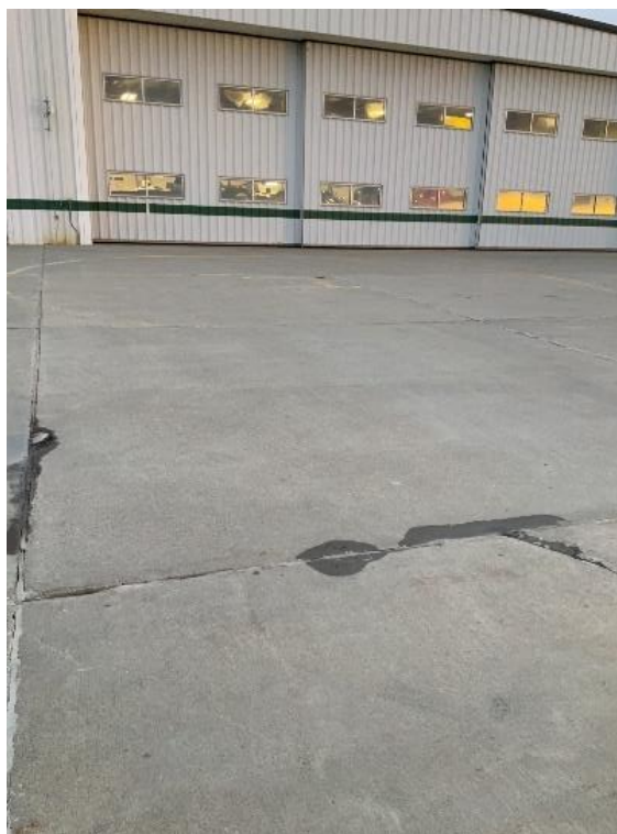
Joint damage and faulting on concrete helipads
